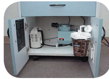
Pump compartment located in base of cabinet
